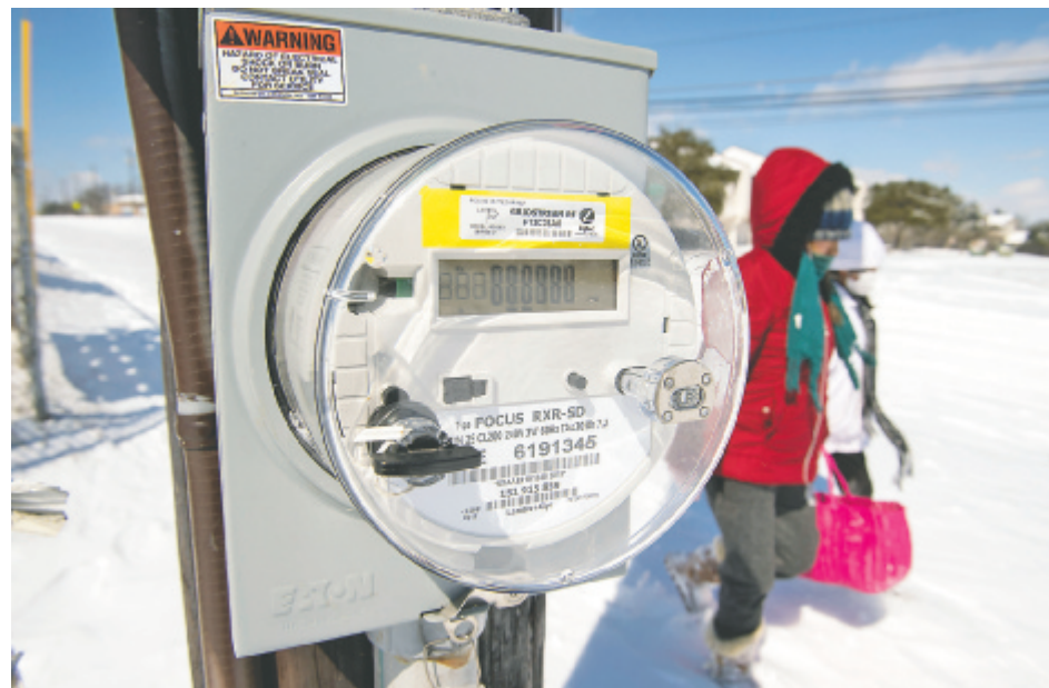
An electric meter in North Austin on February 15, 2021, following Winter Storm Uri
